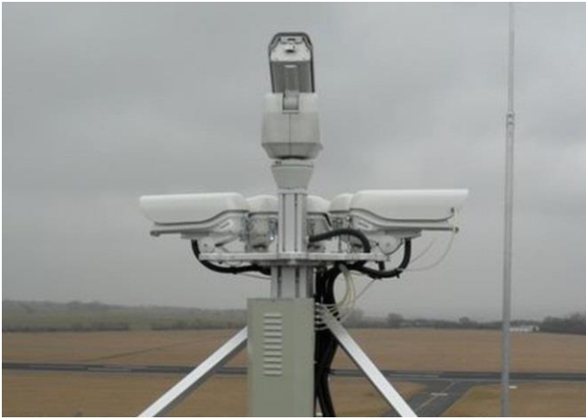
Figure 3. Camera on the top of Erfurt-Weimar Tower.
